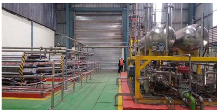
INSTALLED HYDROGEN PLANT · STACKS AND BALANCE OF PLANT
