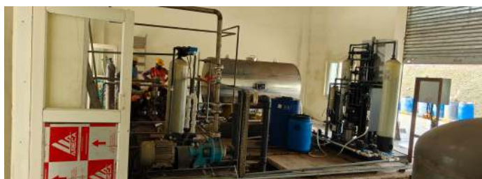
WATER TREATMENT AND UTILITY SKID
