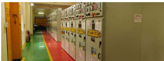
ELECTRICAL AND CONTROL ROOM · INSTALLED PROJECT
