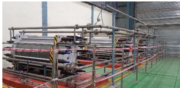
INSTALLED ALKALINE STACKS
